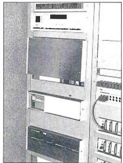
A separate microprocessor and floppy disc input for the automation system is installed in the technical area.
